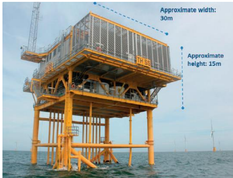
Figure 29: An example of an offshore HVAC Substation [32]
