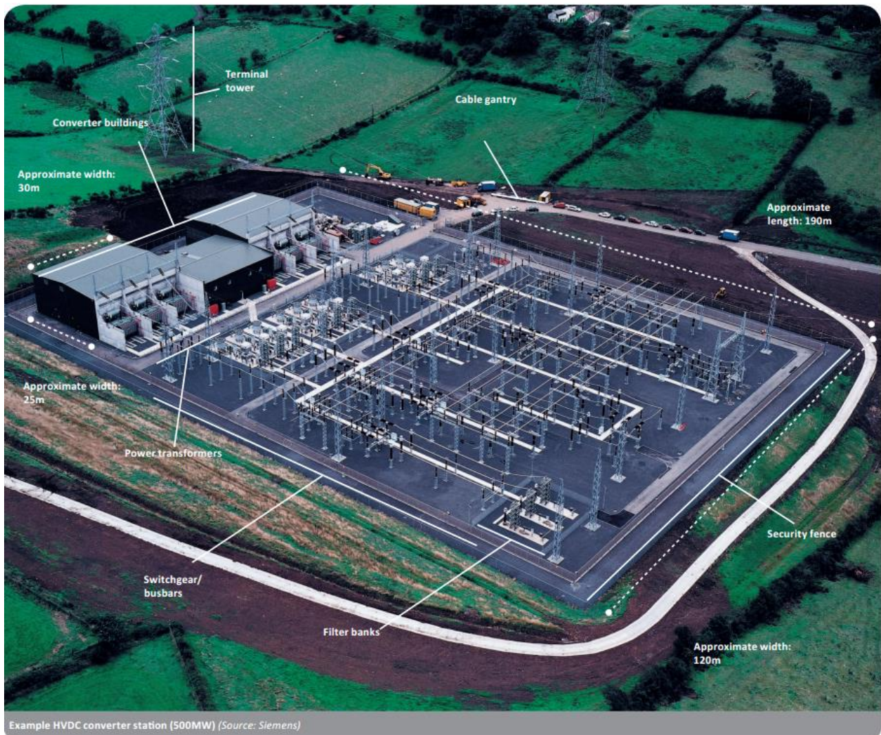
Figure 34: An example onshore HVDC converter station [32]
