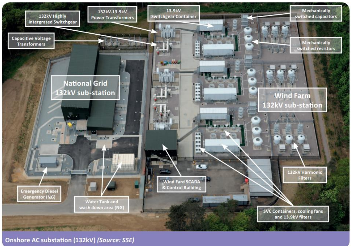
Figure 35: An example onshore HVAC substation [32]
